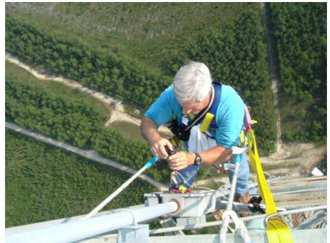
Paul Magnabosco installing the electrical tie-in for the CARES Repeater 1000 feet up the antenna tower.
